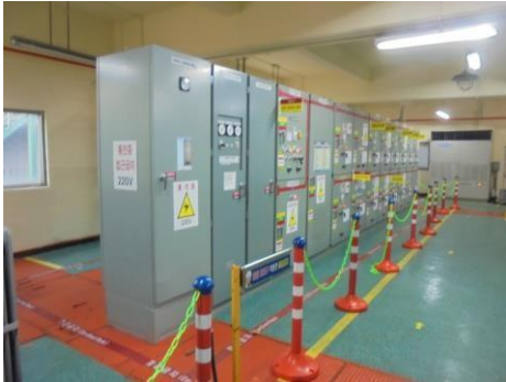
Block power supply(VCB, ACB) And prohibit arbitrary operation
